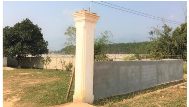
Fence construction of Kokmouang Health Centre in Kokmouang Village, Sing District, Luang Namtha Province by community contribution and it completed on 18 February 2021
